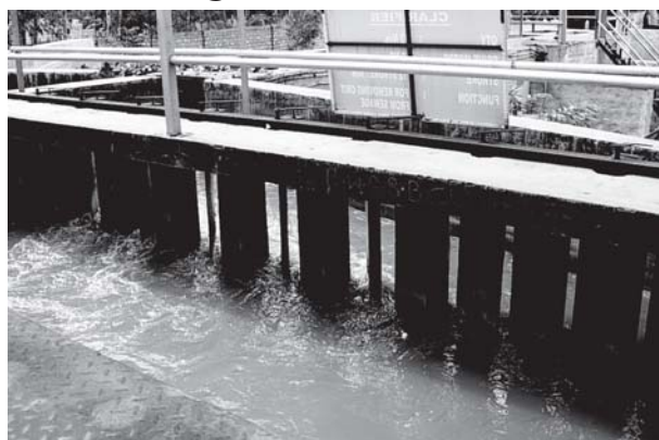
Fig. 18.4 Grit and sand removal tank
